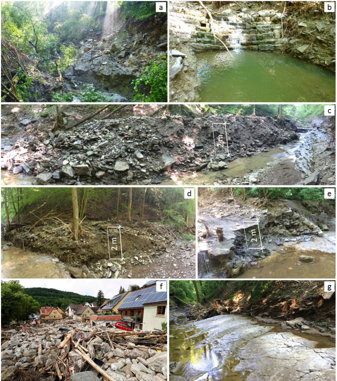
FIGURE 3.6: Erosion in the Orlacher Bach (as of 23 June 2016). a. View of landslide number 9 (Figure 3.7) taken from the main body of landslide number 8. b. Intact flow-control structure, which was installed in the early 20th century. c. Right bank along valley section 1, downcutting is >2 m down to bedrock. Incised former fill is poorly sorted, cobbly, and angular. d. Left bank along valley section 1, downcutting is 0.5 to 1.5 m. e. Left bank along valley section 3, downcutting is \sim 1.5 m. Flow-control structure is entirely removed. f. Tree trunks on the Orlacher Street (photo by Kai Pfaffenbach; Sim, 2016). g. Bedrock (Upper Muschelkalk) outcrop in valley section 3.
