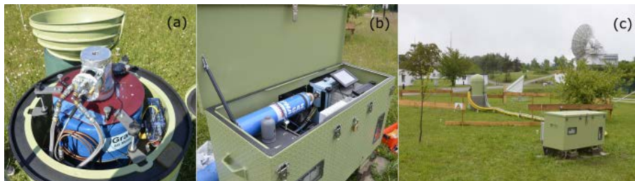
Figure 3.2: Photographs of the gravimeter monitoring system with (a) the iGrav inside the iGFE field enclosure, (b) peripheral hardware inside the iBox, and (c) an overall view of iBox (foreground), dome-shaped iGFE, and the yellow connection hoses. Photos taken on a grassland site of the Geodetic Observatory in Wettzell, Germany.
