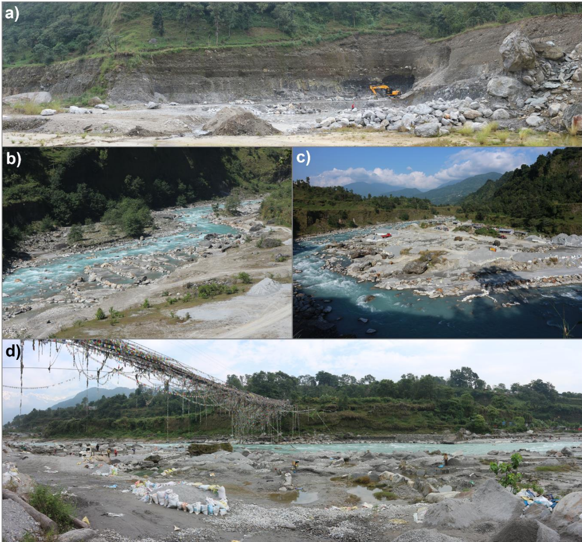
Figure 6.3: Different scales of gravel mining along the Seti Khola. a) Quarrying of gravel beds of the Pokhara Formation near Hemja. b) Groynes built to trap sand carried as suspended sediment load in the upper Seti Khola near Chaura. c) Gravel mining on a point bar near Ghachok. d) Heaps of material extracted from the Seti Khola's bed at Yamdi.
