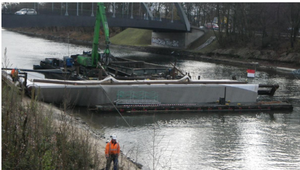
Fig.4.3 Photo of the Nedlitzer Durchstich showing the ongoing construction work at 12.12.2013. Note that at the southern canal bank the old, clogged armourstones were already removed, a geotextile was placed at the channel bottom and that the new armourstones were still missing. The new armourstones were placed and canal bank reconstruction was finished between 12.12.2013 and 01.03.2014 (photo by Matthias Munz).
