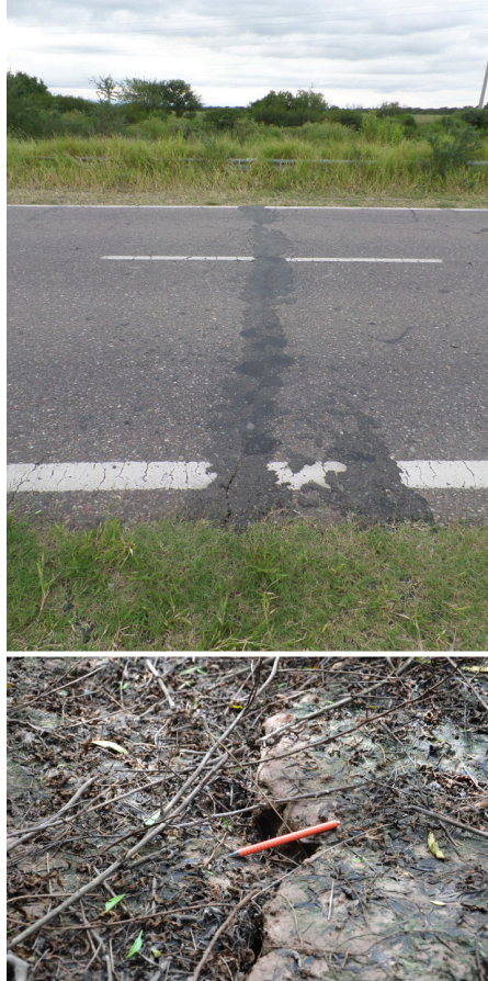
Figure 1.6: Superficial cracks in the epicenter region. Top : Crack at the national road rupturing the asphalt perpendicularly. Facing south. Dislocation crack was already remodeled. Lower : Surface crack close to a hot spring; facing north. Along several tens of meters, a vertical offset in cm-range could be traced.
