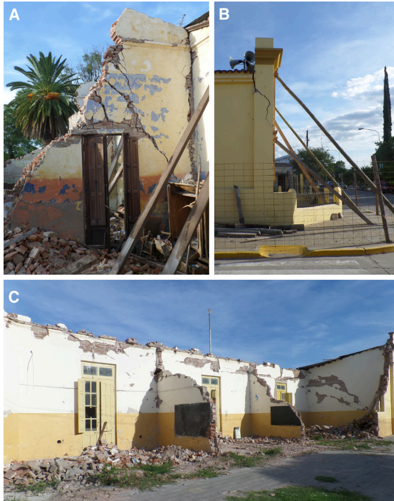
Figure 1.5: Images of destruction patterns in El Galpón I took five months after the earthquake. Image A: Facing north. The west-facing wall collapsed to the left, while the perpendicular wall shows crack patterns related to the extensional forcing. Image B: Facing south. The western wall tilts towards the west and is supported by wooden planks against further damage. Image C: Facing southeast. It shows the former school building where the western wall and the roof collapsed.
