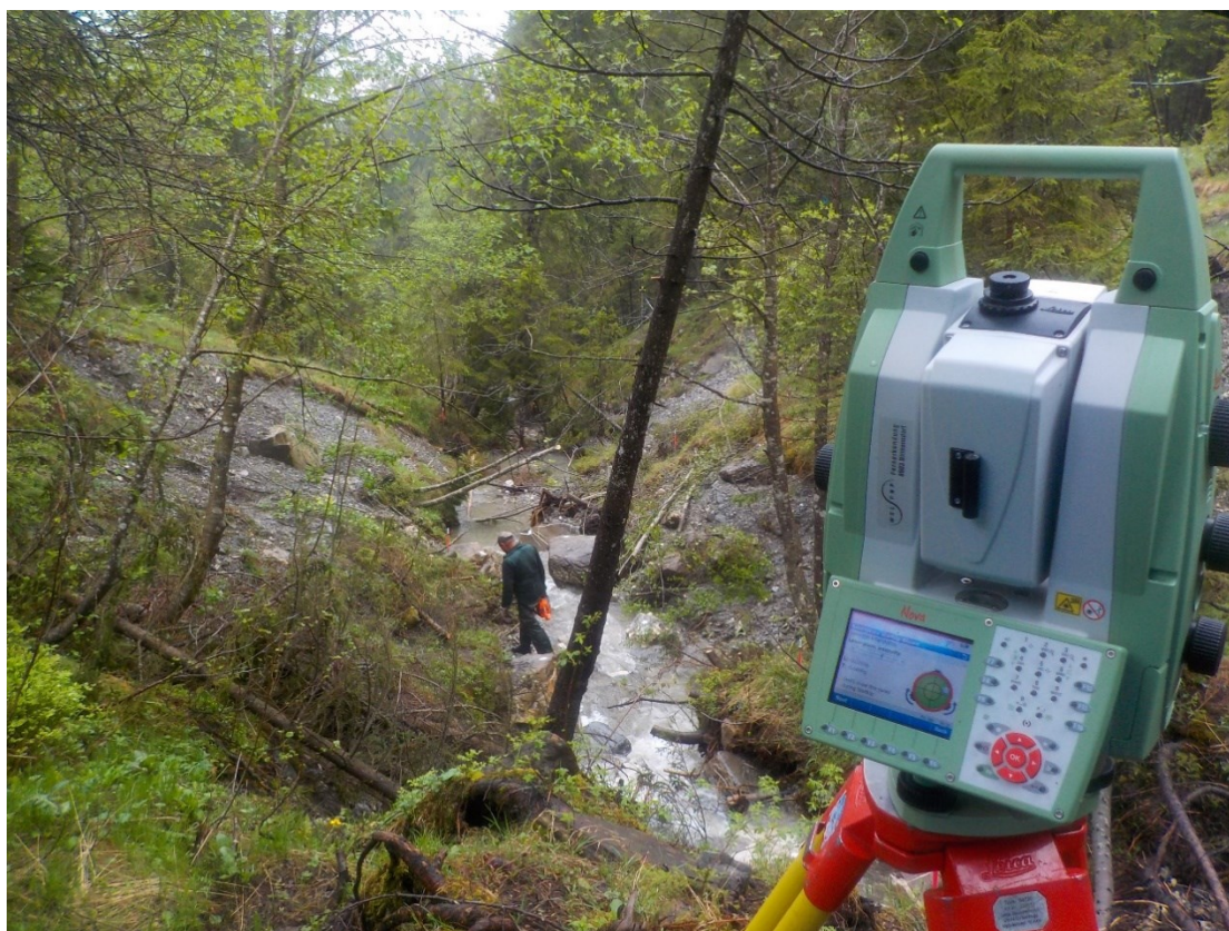
Fig. 10: During a field survey of the long profile the total station (right) is setup with known coordinates and orientation. Then, single point measurements to a reflector held by an assistant in the channel bed are performed. A usual long profile survey of the 550 m study reach consists of ~1000 single point measurements surveyed over a period of three days.
