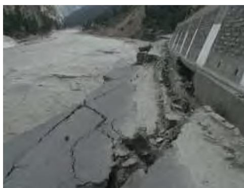
Figure 18: Picture showing damage to roads
