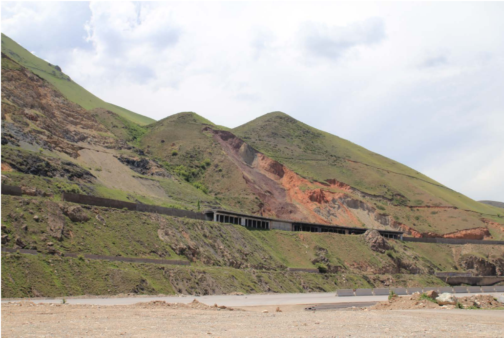
Figure 1: Landslide threatening the main and only railroad between Bishkek and Balykchi (NW Issyk Kul).
